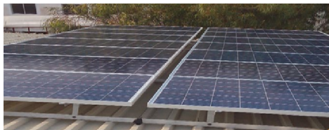
South Sudan: Solar panels installed at the public health lab
